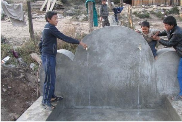
The new water taps at the washing place..
